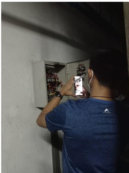
Gambar 3. Instalasi Box Panel
